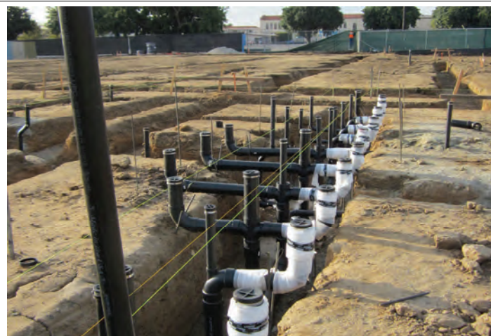
Building Underground Plumbing
