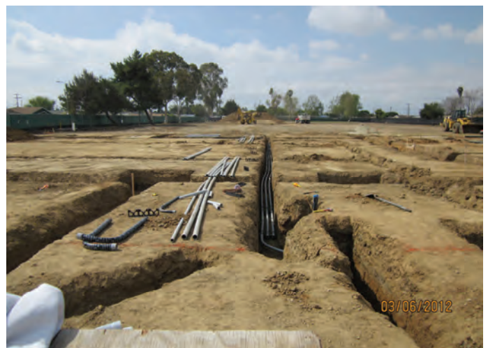
Underground Electrical Piping
