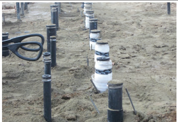
Building Underground Plumbing
