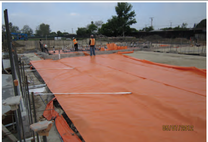
Methane Mitigation System (Remaining Areas)
