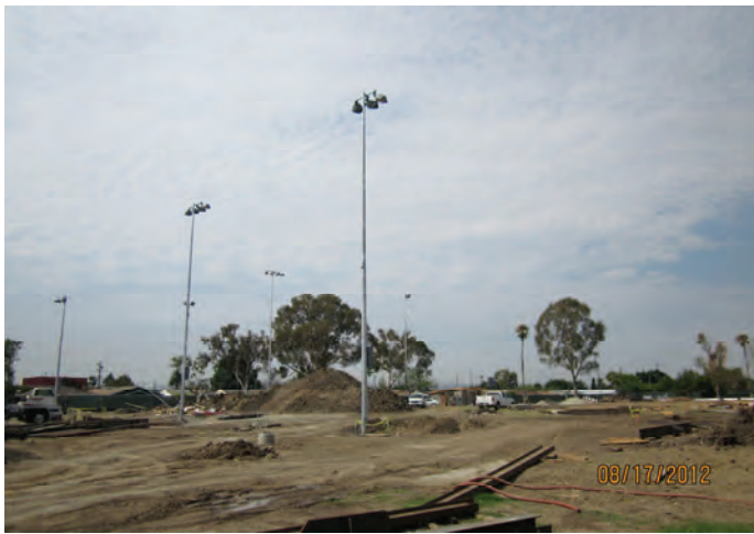
Musco Lights Installed
