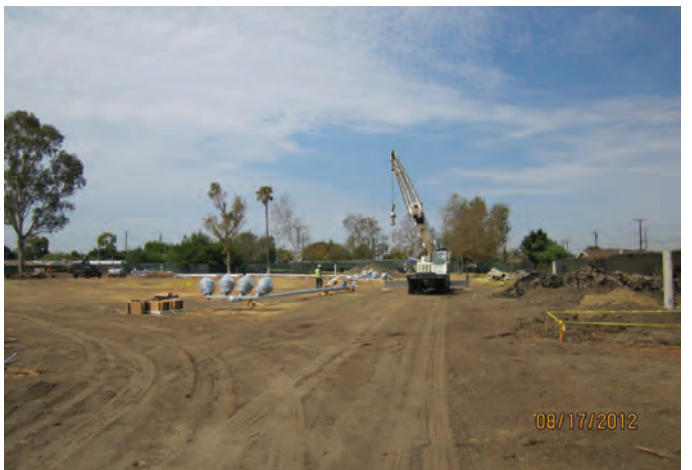
Musco Lights (Ready for Installation)
