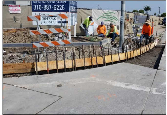
Powell forms curb and gutter at north west corner of Carson St.
