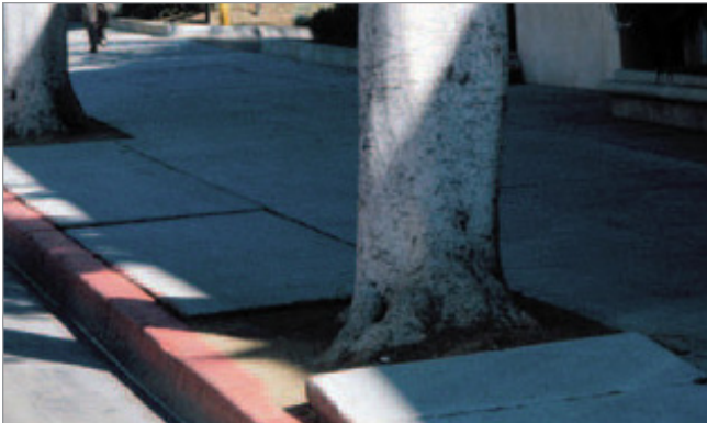
Because the soil under a concrete sidewalk is extremely compacted, the roots remain in the tree well and the tree becomes rootbound.
