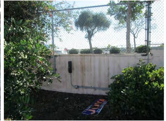
15. Wall along southern Site boundary with apparent power related source.
