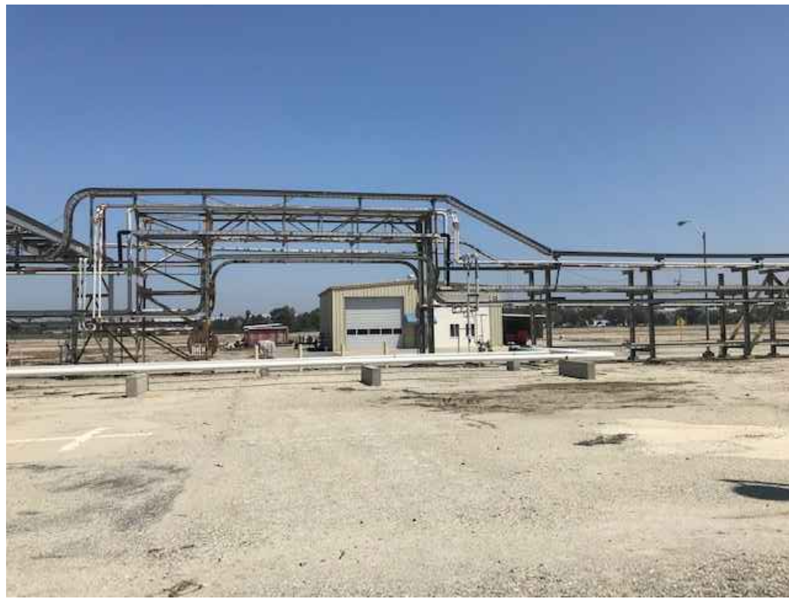
4 EXISTING EAST/WEST PIPE RACK THAT WILL CONVEY THE 4-INCH NATURAL GAS LINE, VIEW NORTH
