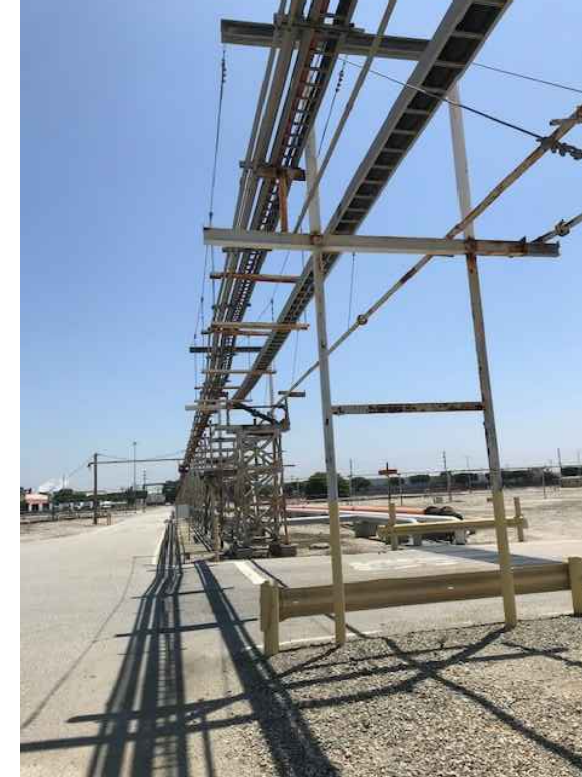
3 EXISTING DRIVEWAY CROSSING IN A PRECAST TRENCH WITH GRATE COVERING, VIEW EAST
