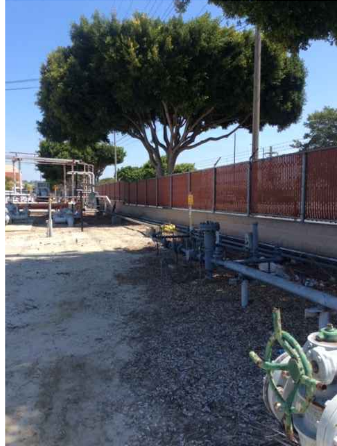
1 APPROXIMATE LOCATION OF CONNECTION TO SOCAL NATURAL GAS MAIN NEAR WILMINGTON, VIEW NORTH
