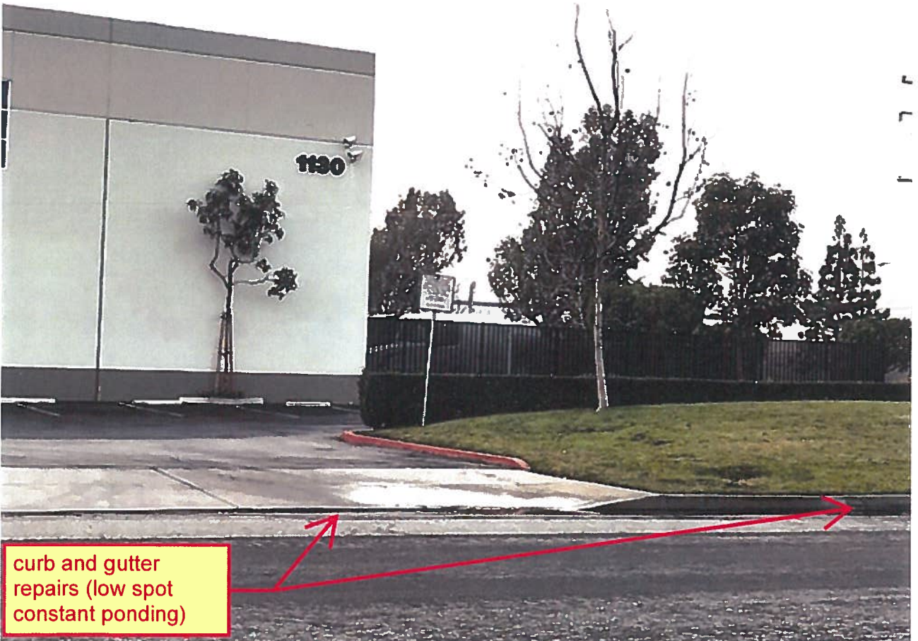
Pavement repairs needed at street
