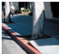
2. Because the soil under a concrete sidewalk is extremely compacted, the roots remain in the tree well and the tree becomes rootbound. The only place the roots can escape the tree well is between the soil and concrete, resulting in uplifted sidewalks. The uplifting is more pronounced for Ficus trees because they naturally have roots that grow on the surface.
