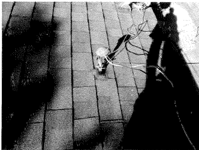
The rear house cable feed support has come loose. Cables are laying on roof.
