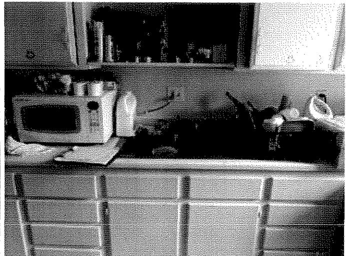
Rear house: I was not able to inspect counter tops due to dishes and stored items.
