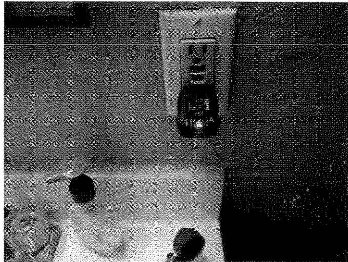
Open grounds noted in the "rear house" bathroom.
