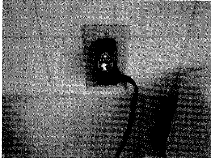
GFCI did not respond to test. Front house
