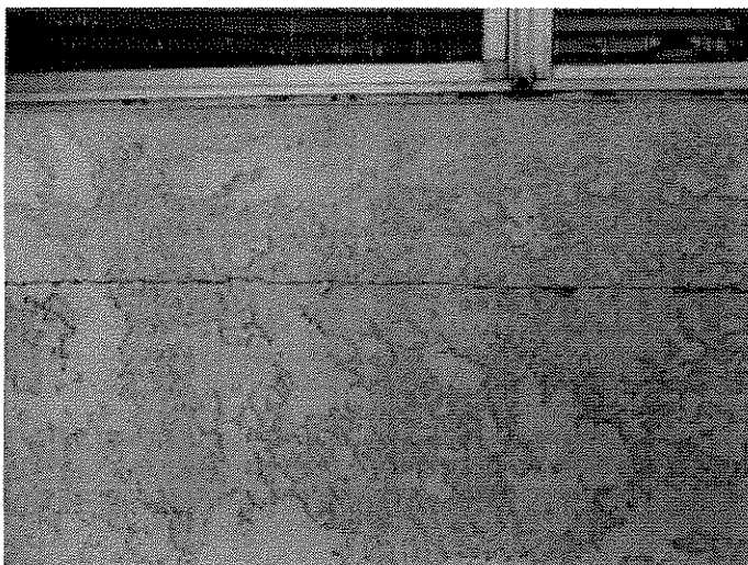
Some cracks noted in stucco.
