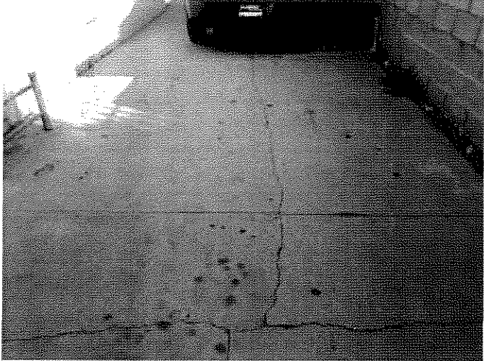
Cracks noted in driveway.
