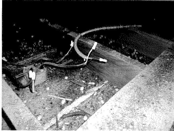
Splices made outside of j-box, front house.
