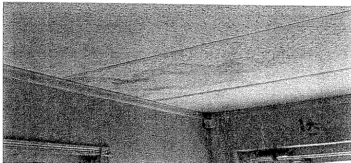
ROOF LEAK OBSERVED AT S/W & S/E CORNERS OF SHOW ROOM (REFER TO ROOFER)
