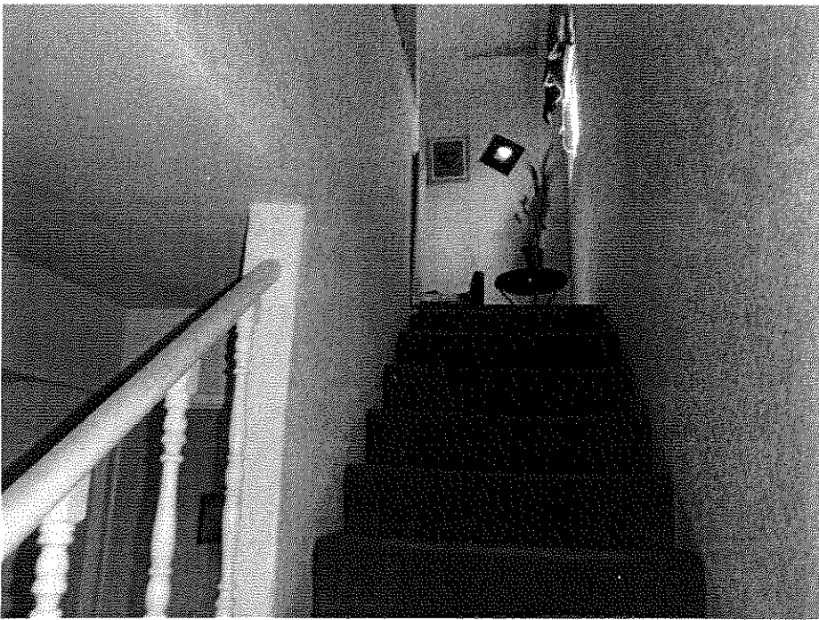
Figure 8-no handrail at the top section of the stairway
