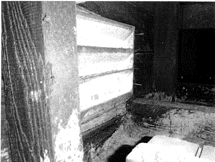
Figure 10-one the many damaged/missing attic ventilation screens
