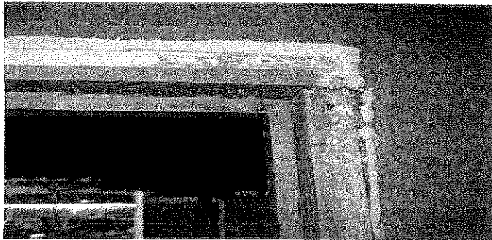
MOLDING MISSING AT DOOR JAMB IN LUNCH AREA (REFER TO CARPENTER)
