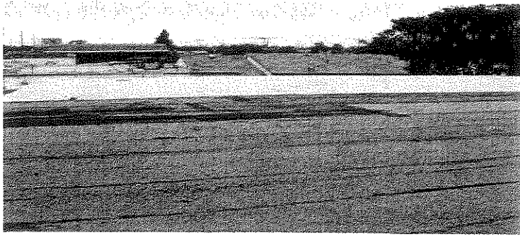
ROOF LEAKS IN SEVERAL PLACES (REFER TO ROOFING CONTRACTOR)
