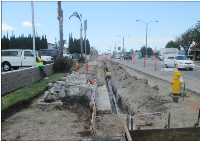
Electrical Lines at CVS
