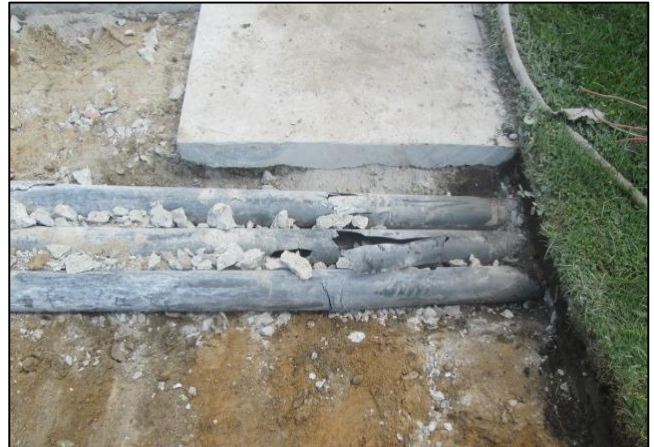
At CVS Sidewalk Drain Lines Not Shown on DWG
