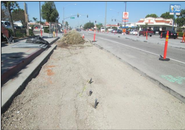
Electrical Conduit and Irrigation Line
