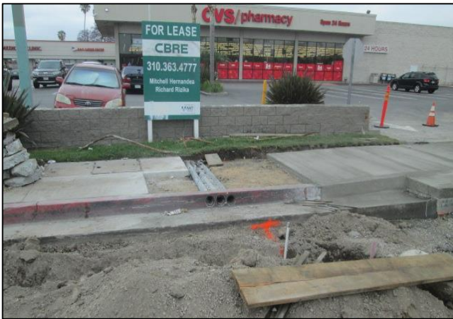
Existing Drain Lines to be Replaced
