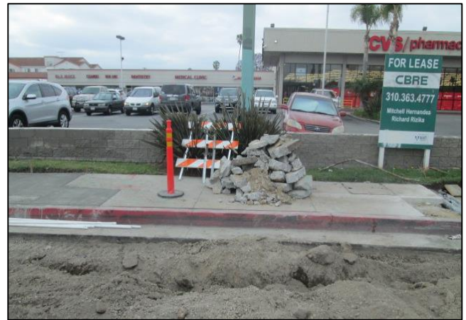
Rubble to be Removed
