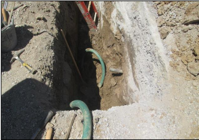
Cal Water Working in a 6' Deep Trench No Shoring
