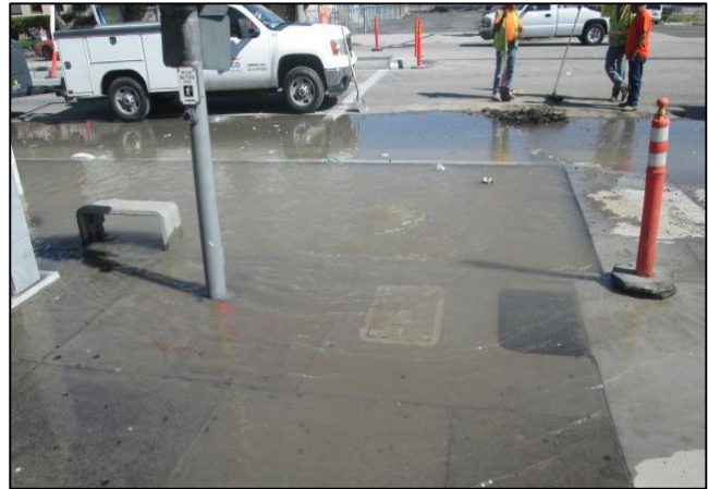
Results from Broken Water Service Line
