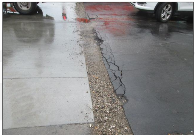
AC Needing Repair
