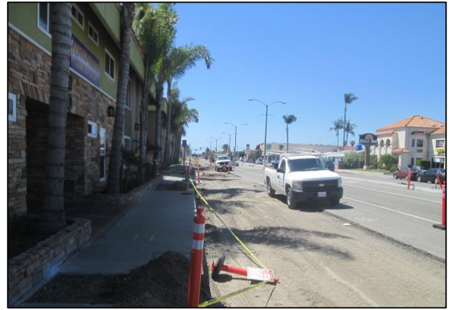
Delineators Require House Keeping
