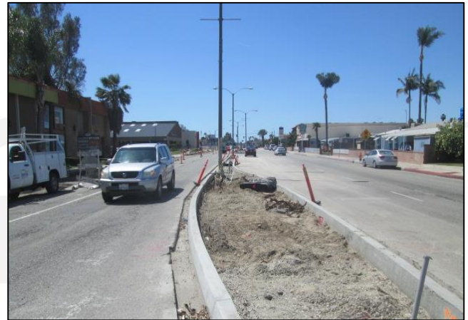
Slot Cut that Requires Delineation
