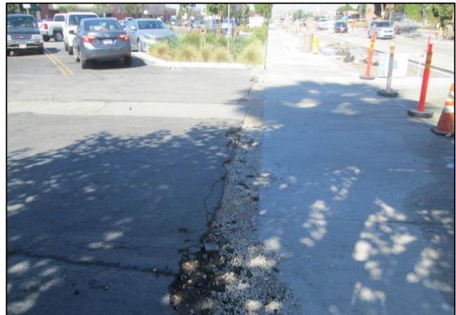
AC Requires Repair
