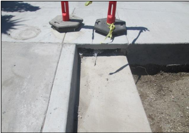
Typical Blockage in New Culvert
