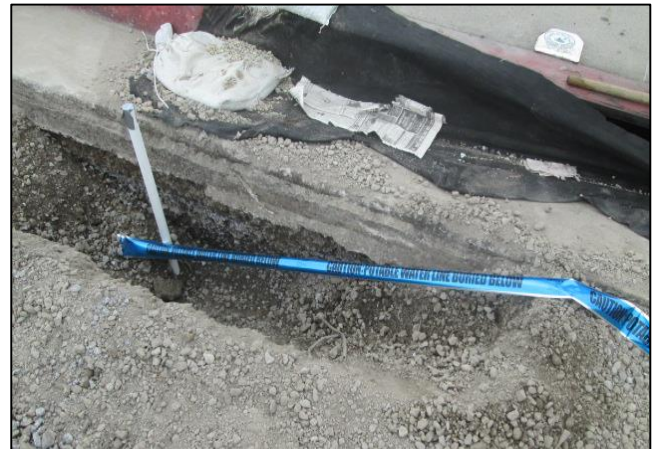
Potable Water with Warning Tape
