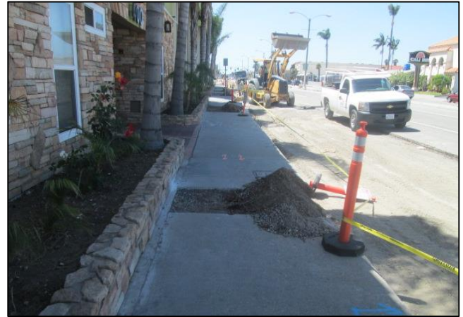
Open to Peds Sidewalk Requires Delineation and Caution Tape
