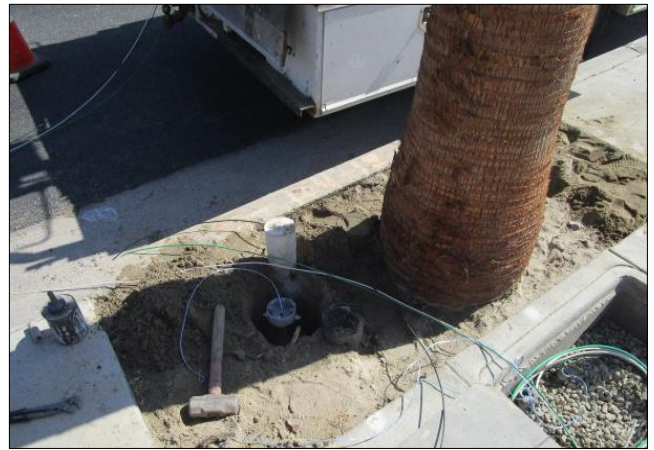
Wiring palm tree uplights.
