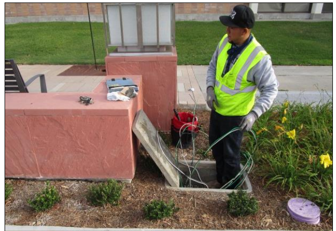
Wiring plinth lantern east of Main.
