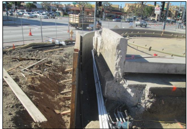
City Hall Fountain Skimmer Lines
