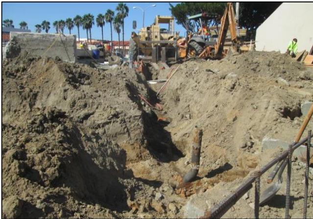
Clogged Drain Replacement at City Hall
