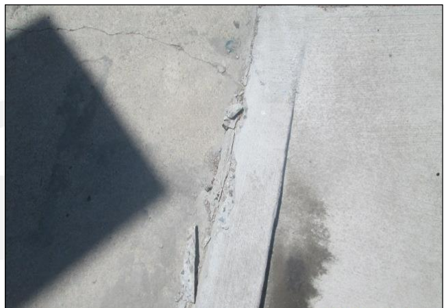
Broken ADA Curb at Grace and Carson
