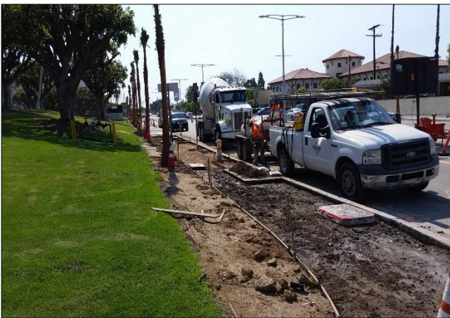
National Ready mix arrives for Portland Cement Concrete (PCC) west bound Carson.
