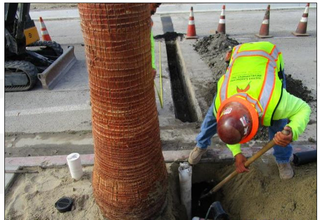
Connecting irrigation mainline crossing Carson.
