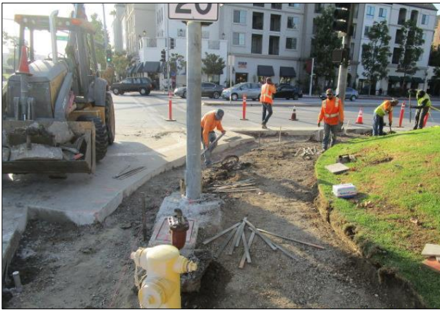
Grading and compacting for curb ramp south west corner of Carson and Avalon.
