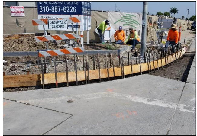
Powell forms curb and gutter at north west corner of Carson St.
