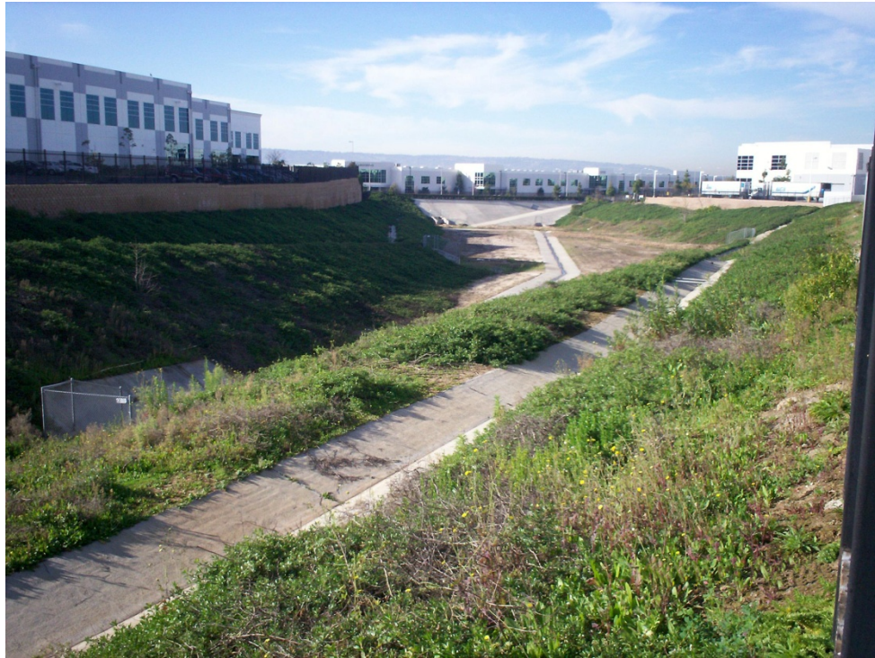
Photo 3: Stormwater basin, facing southwest at fence along driveway of 18030 Bishop Avenue (approximate address)
