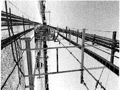
3 EXISTING DRIVEWAY CROSSING IN A PRECAST TRENCH WITH GRANITE COVERING, VIEW EAST
